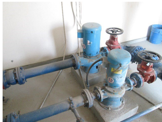
Fairview Heights Booster Pump Station.
