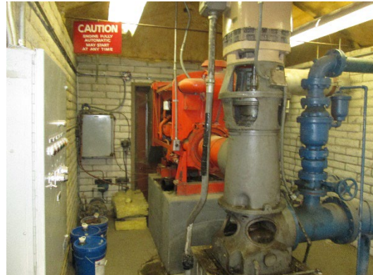
Well No. 4 diesel pump motor and well pump.
